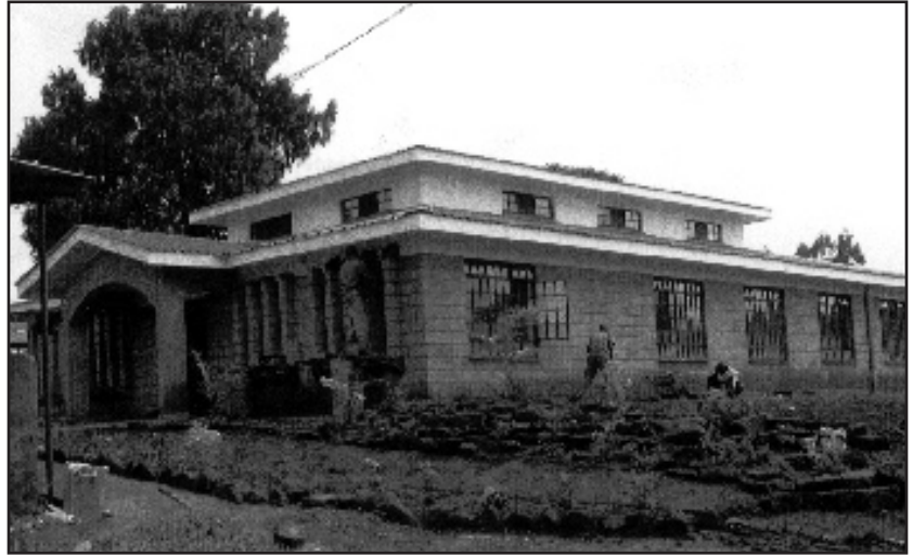
Construction workers putting the final touches on the dental clinic in Kikuyu, Kenya.
